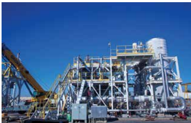
Figure 2. Nikkiso Cryo cryogenic pump test facility.
